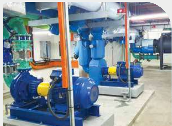
The newly installed fourth chiller in the plant room.
